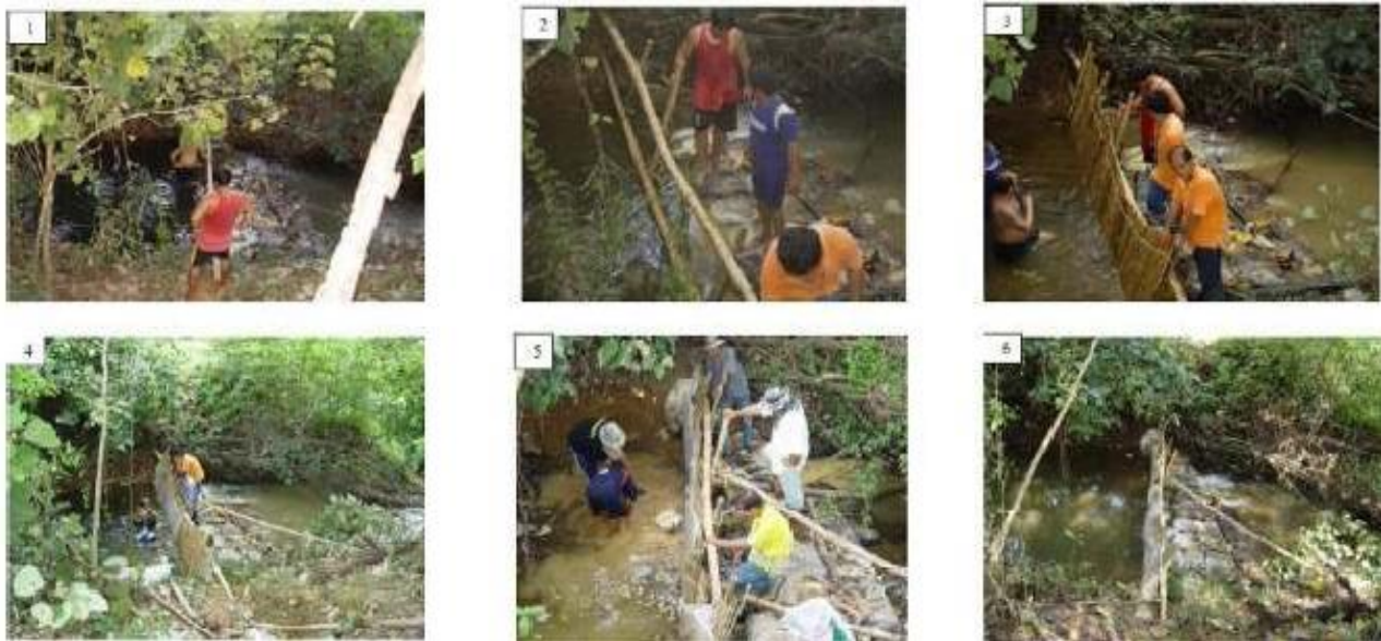
Fig. 1 Step of making low cost check dam with local material utilization following
